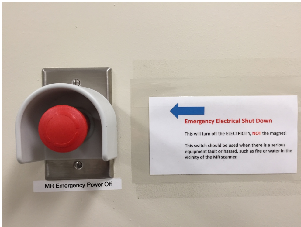
FIGURE 3 THE EMERGENCY POWER OFF BUTTON IN THE CONTROL ROOM.
