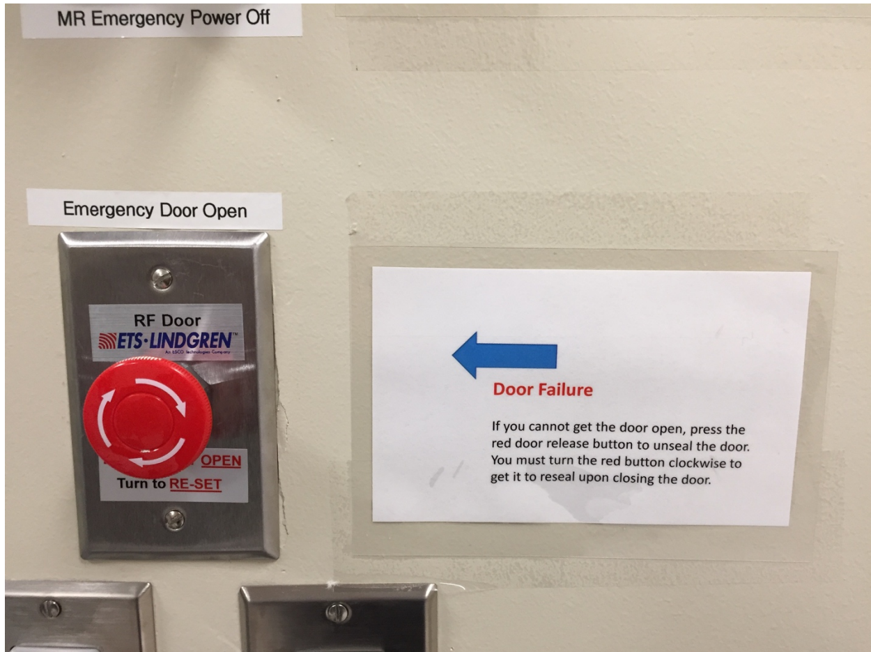
FIGURE 5 EMERGENCY MAGNET ROOM DOOR OPEN BUTTON IN THE CONTROL ROOM.
